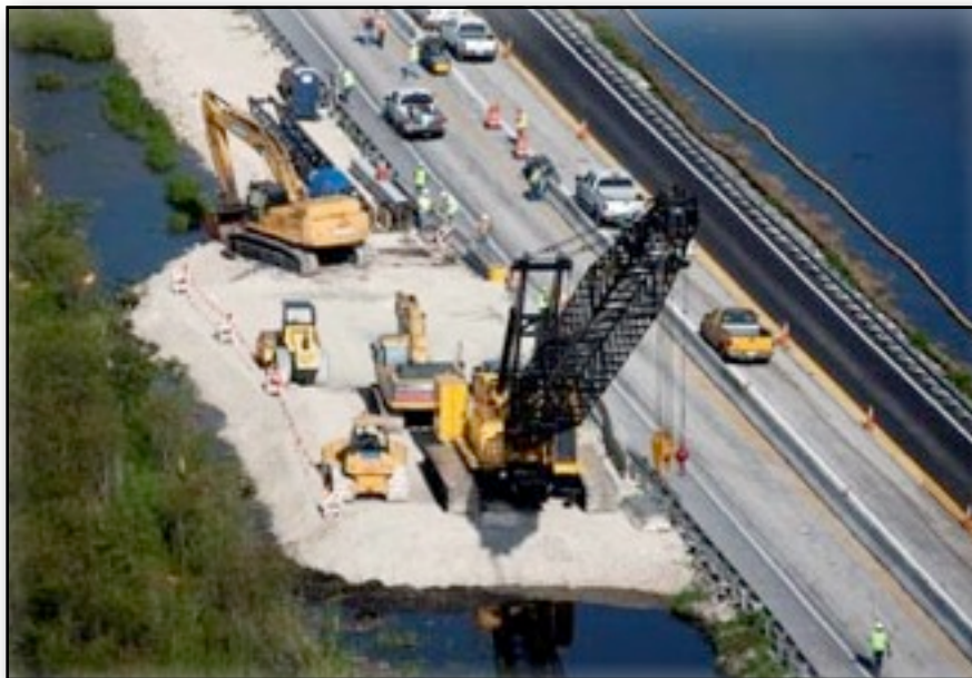
Construction on the Tamiami Bridge project. Photo from U.S. Army Corps of Engineers.
